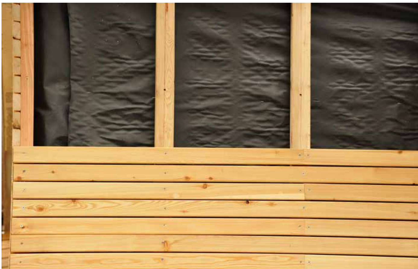
Installation of Raute profile 28 x 68 mm, ventilated facade with the use of diffusion foil
